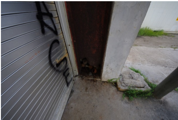
Rusted Piers on Existing Warehouse
