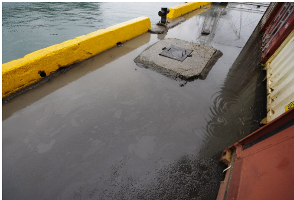
Water Pooling on main wharf
