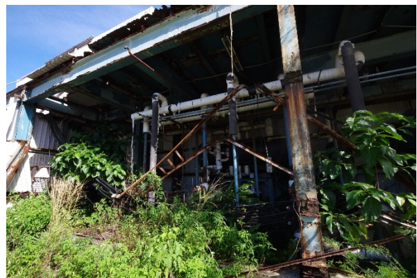
Derelict Fresh Tuna Incorporation Building
