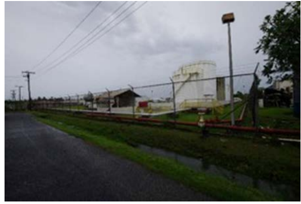
Fuel Storage Area
