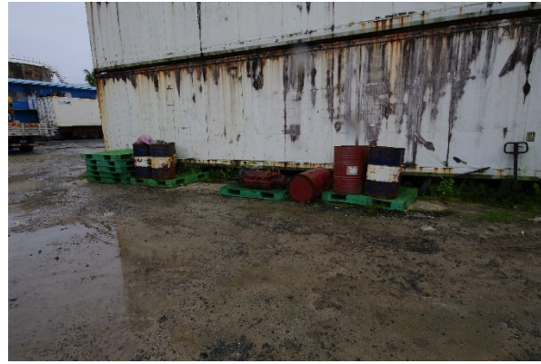
Water Pooling in the Container Yard
