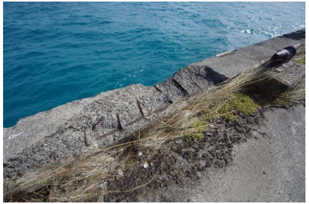
Damaged Wharf Frontage
