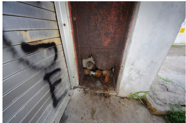
Rusted Piers on Existing Warehouse
