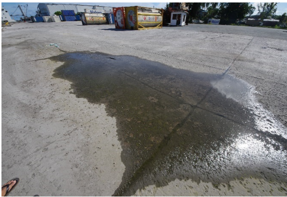
Water pooling following rain
